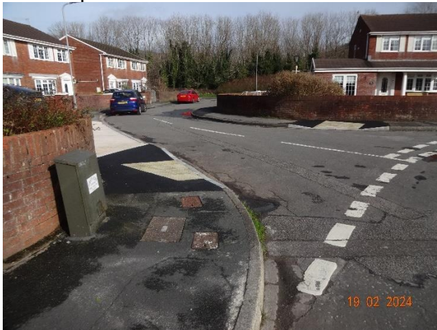
Figure 6: Example of a new dropped kerb and tactiles installed near to Village Road.
