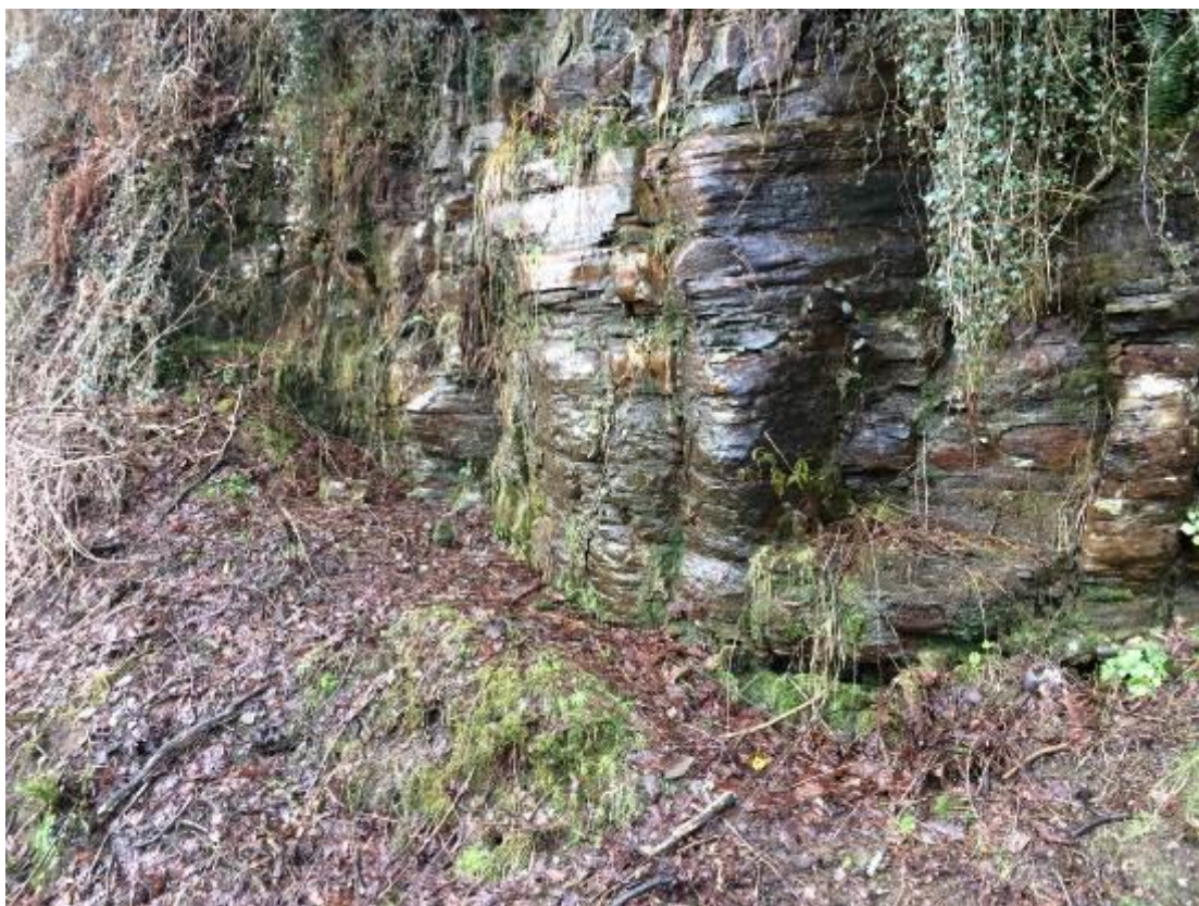
Photograph 22 – Moderate seepage from cliff face
