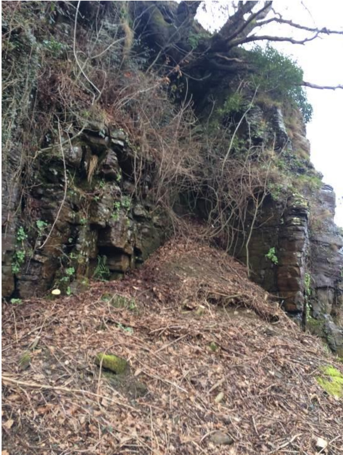
Photograph 23 – Slumping of debris from crest to toe
