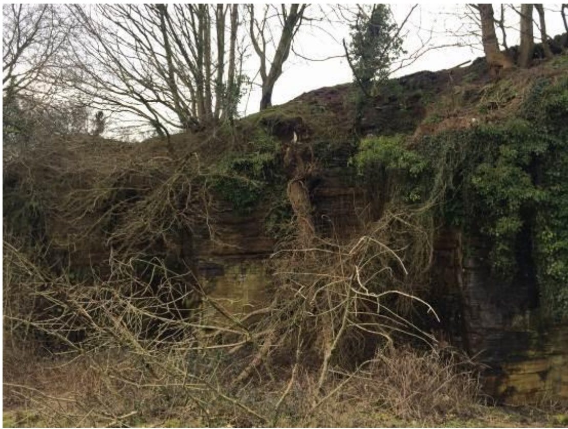
Photograph 6 – Fallen trees at crest of high wall
