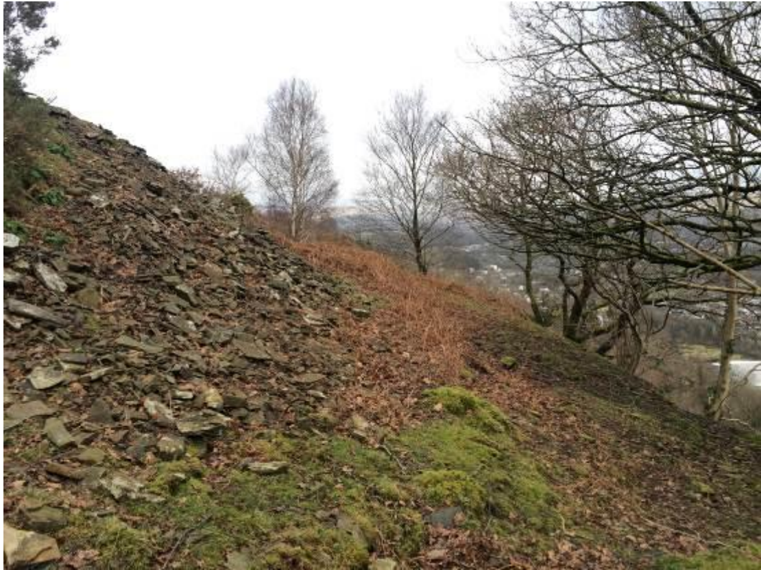
Photograph 13 – Toe of spoil mound along cliff edge
