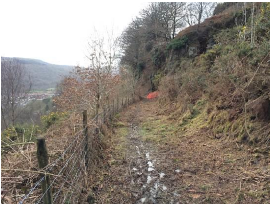
Photograph 20 – Surface water flows disappearing to ground
