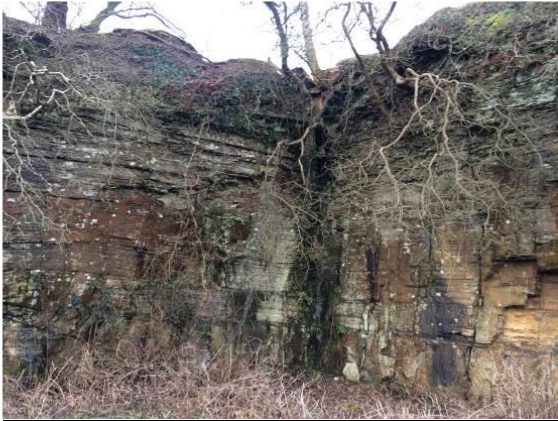
Photograph 3 – Quarry high wall showing seepages
