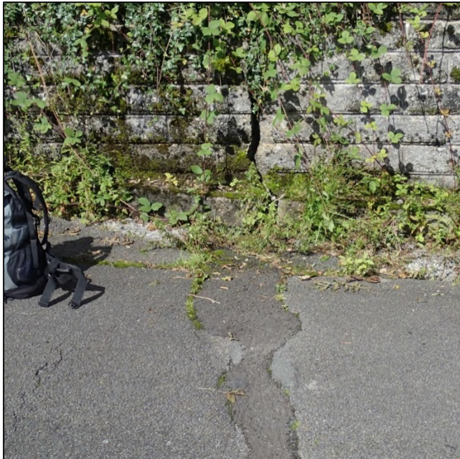
Insert 36 - 20mm tensional opening in retaining wall with distress continuing across Graig Road (15/8/17)
