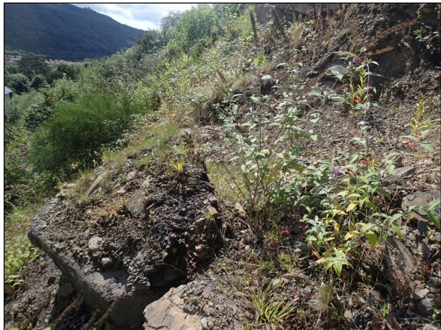
Insert 40 - Tension crack behind block exposed block of sandstone in are modified following the 2012 landslide (15/8/17)
