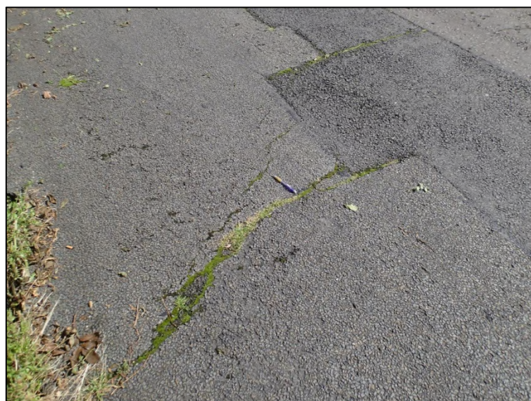
Insert 37 - Left stepping en-echelon distress in Graig Road crossing recent repairs (15/8/17)
