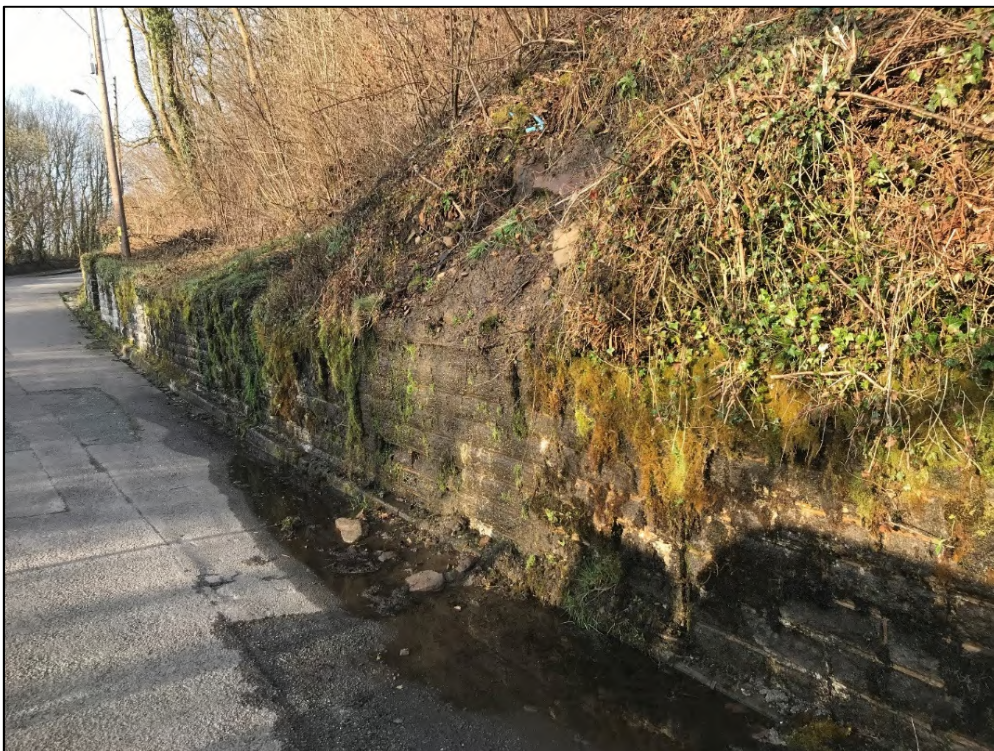
Insert 1 Photograph showing area of excess surface water on the northern retaining wall of Graig Road. Colluvium present on top of the retaining wall. Photograph taken looking south-west on 9 th April 2018.
