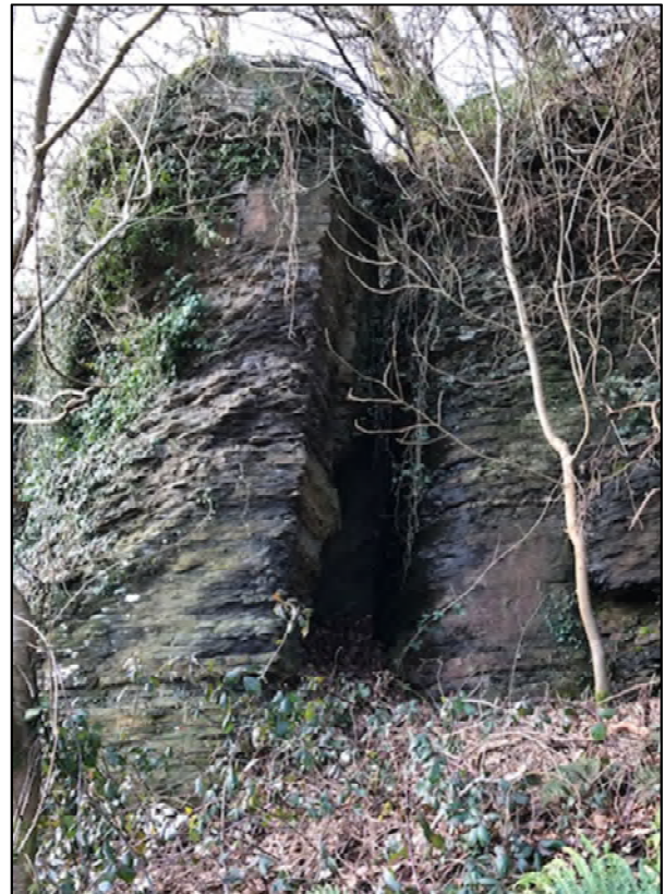
Insert 4 - Potential rock fall block along cliff-line
