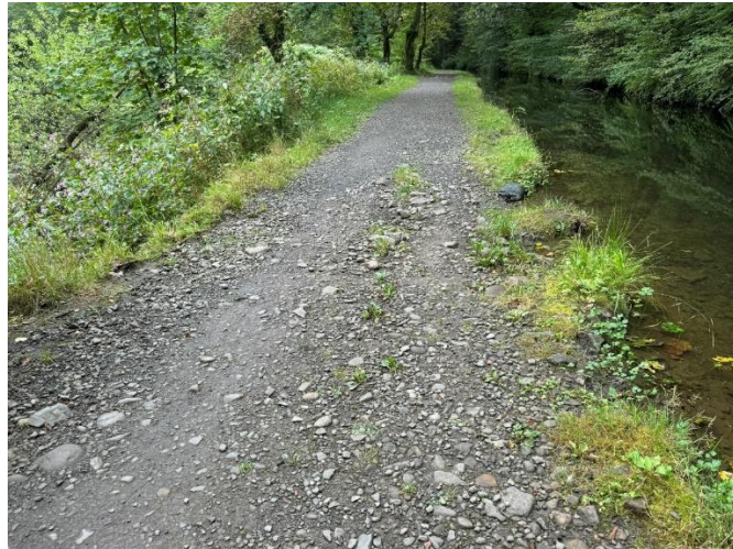
Image 50 - Evidence of overtopping/ flooding (sandbag) across footpath from Canal near Pontygwaith Bridge
