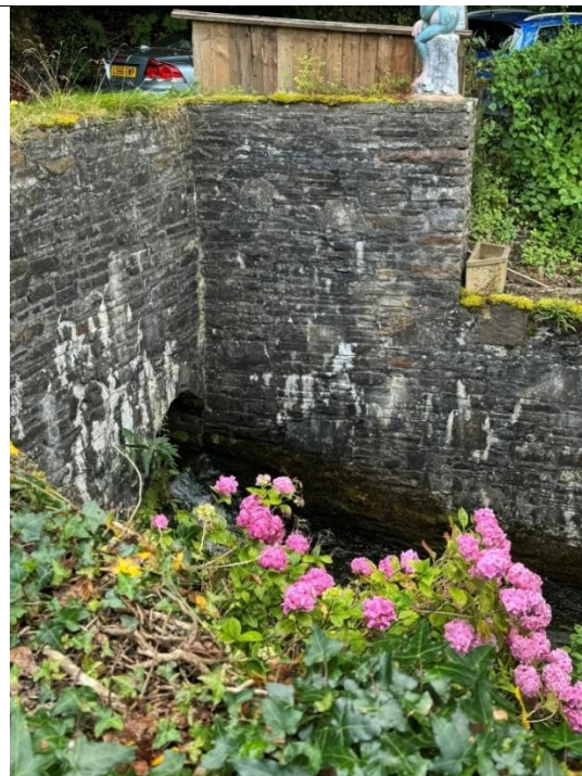
Image 36 – Tonna Lock Structure with efflorescence on bricks and rhododendron growing on embankment
