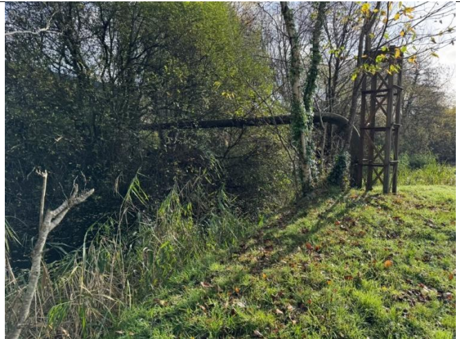
Image 16 – Pipe Bridge with adjacent metal tower. Rusted exterior
