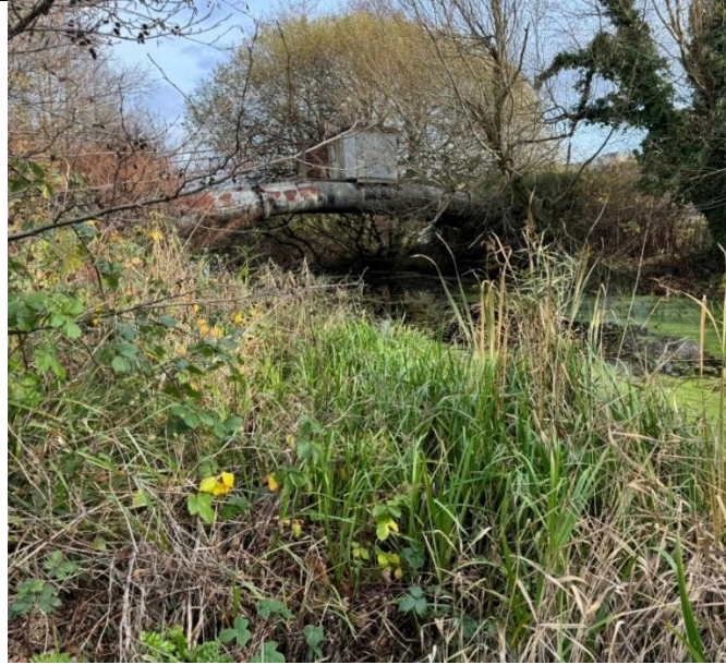
Image 10 – Pipe Bridge with rusted exterior
