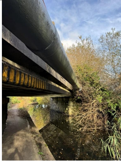
Image 18 – Swansea and Rhondda Bay Railway Bridge with thick vegetation growing on pier
