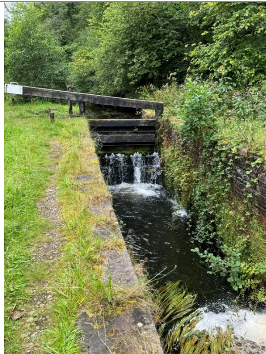
Image 52 - Lock Machin with inoperable lock
