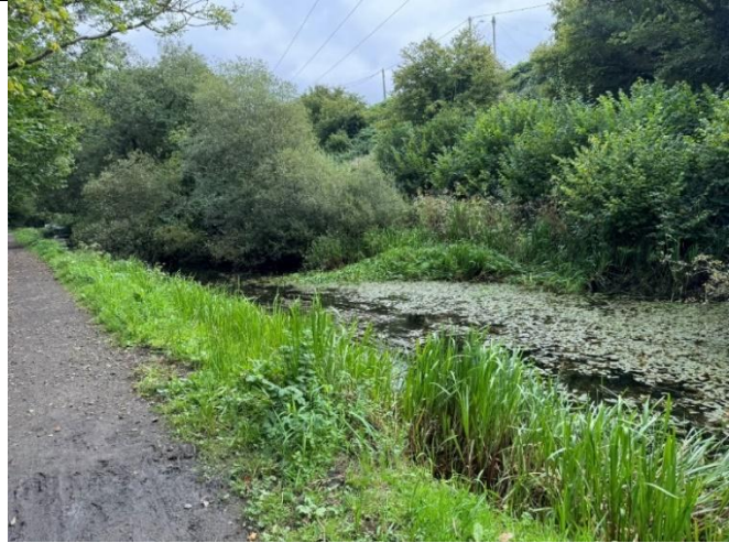
Image 70 – Section of the canal near Ynysbwlllog Aqueduct with reeds and lily pads obstructing navigation
