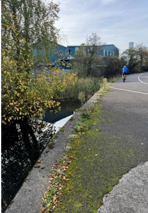
Image 29 – Canal section near Pipe Bridge clogged with reeds and overhanging tree
