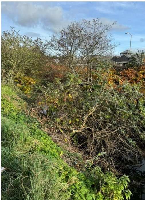
Image 31 – Bridge Street Bridge canal condition with large vegetation and trees overhanging water
