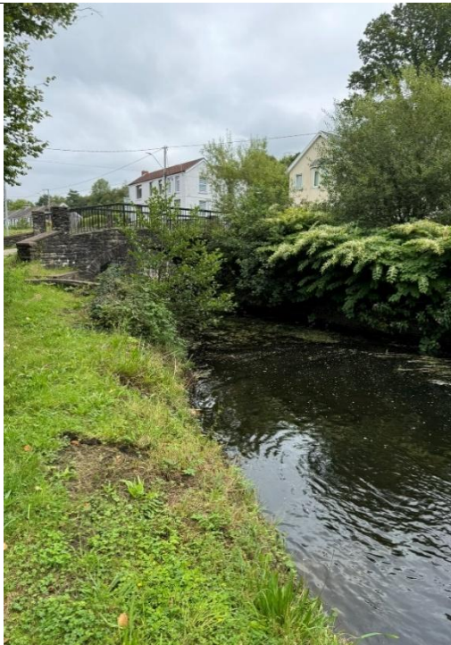
Image 59 – Abertwrch Bridge with vegetation growing next to abutments
