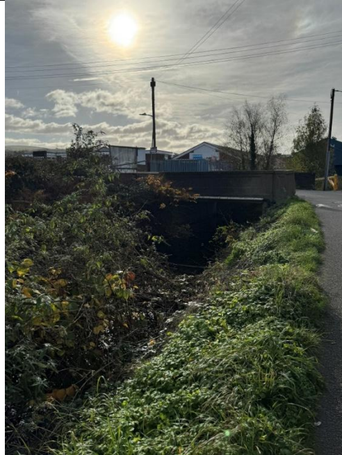
Image 26 – Milland Road Bridge with insufficient headroom for navigation
