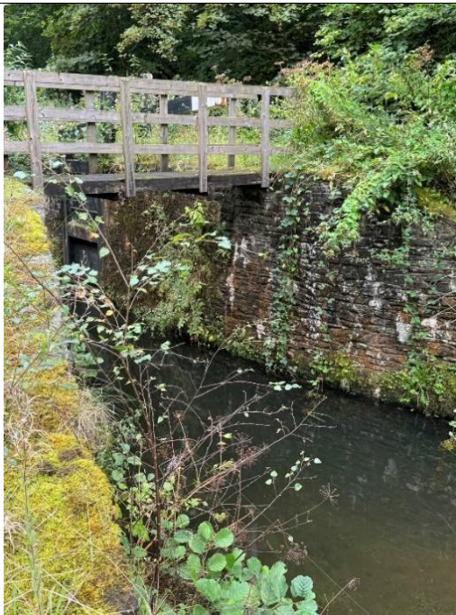
Image 51 – Lock Machin Bridge with buddleia growing on one abutment
