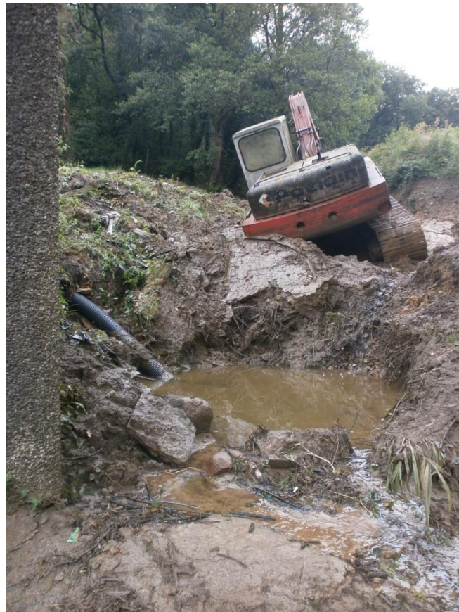
Figure 9, Photograph of the location of culvert (ID: CUL_0427) post flood event
