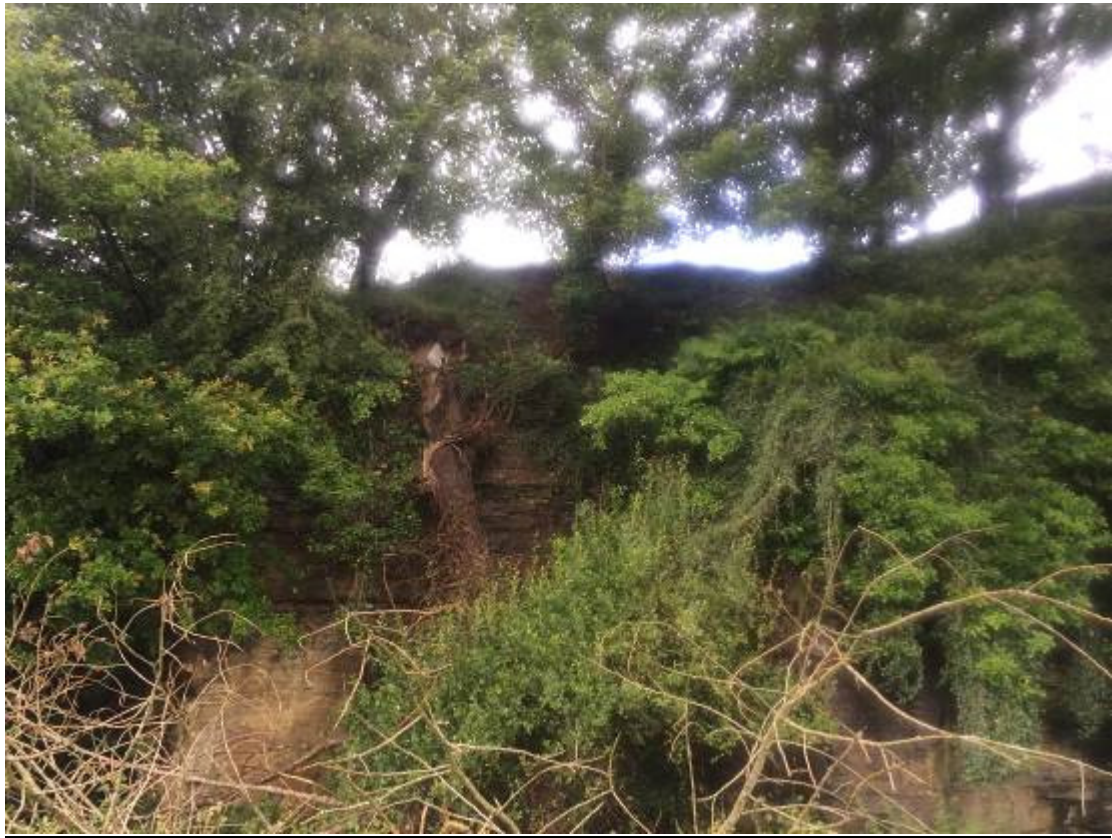
Photograph 3 – Quarry high wall showing fallen trees
