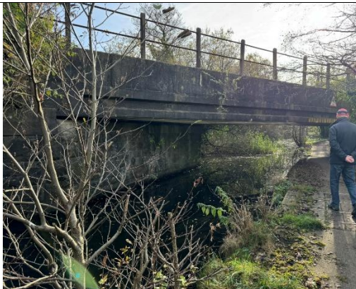
Image 19 - Swansea and Rhondda Bay Railway Bridge with low headroom (5'8) for pedestrians
