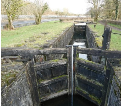
Image 81 – Crugiau Lock now inoperable
