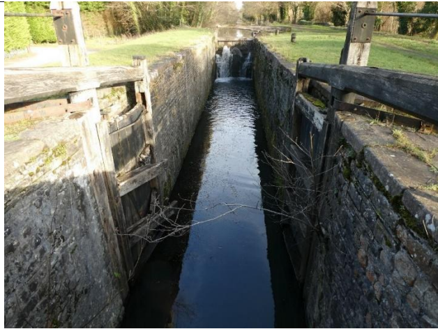
Image 86 - Aberclwyd Lock currently inoperable
