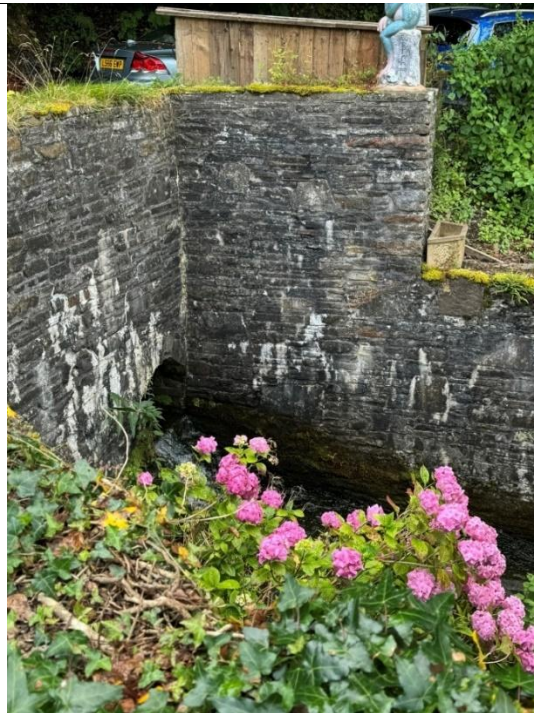
Image 36 – Tonna Lock Structure with efflorescence on bricks and rhododendron growing on embankment
