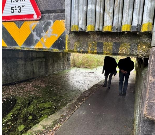
Image 9 - Neath Junction Rail Bridge highlighting low headroom (5'3) for pedestrians but sufficient for canal navigation
