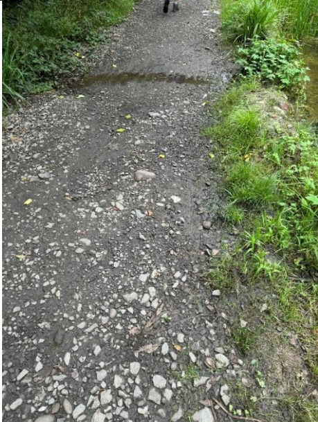
Image 47 – Evidence of overtopping from Canal near Howards Footbridge
