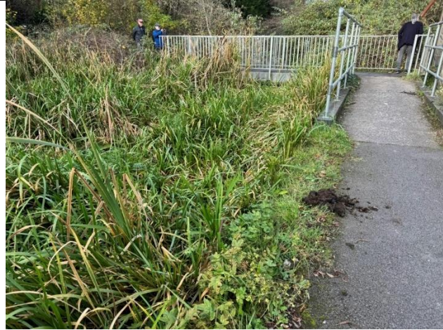
Image 6 – Canal adjacent to Lift Bridge overgrown with thick reeds and vegetation
