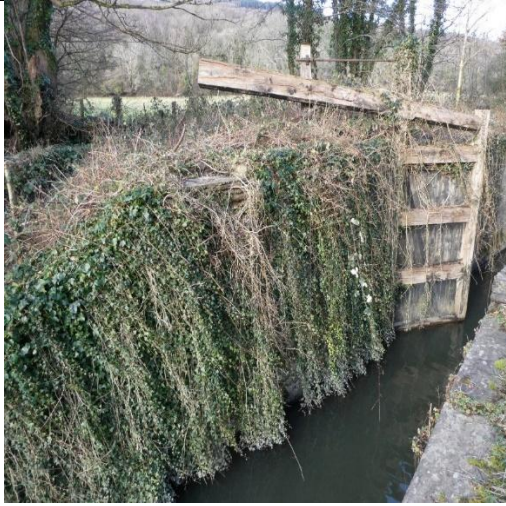
Image 89 - Maesgwyn Lock currently inoperable
