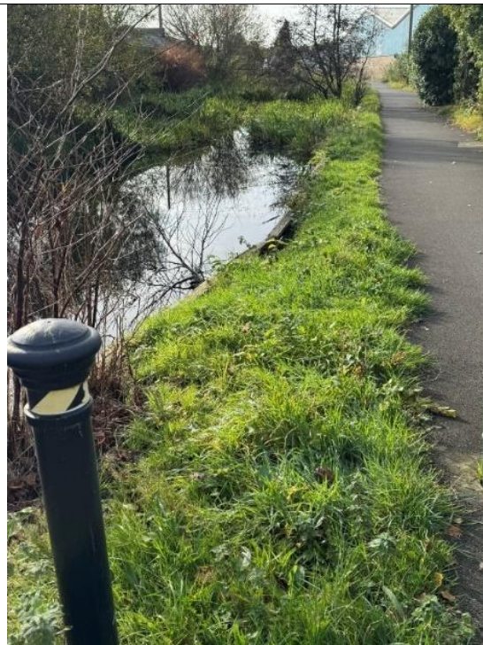
Image 32 – Bridge Street Bridge canal condition with rotten wood supporting canal embankment
