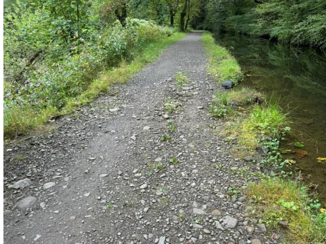
Image 50 - Evidence of overtopping/ flooding (sandbag) across footpath from Canal near Pontygwaith Bridge
