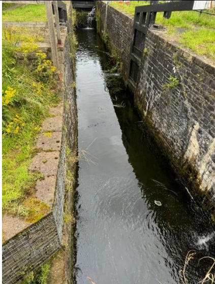
Image 63 – Clun Isaf Lock Structure with efflorescence from masonry
