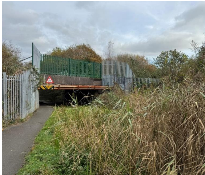
Image 8 – Neath Junction Rail Bridge canal full of thick reed vegetation
