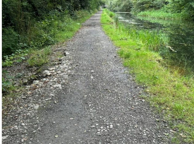
Image 46 – Possible evidence of overtopping (LHS) from Canal near Howards Footbridge
