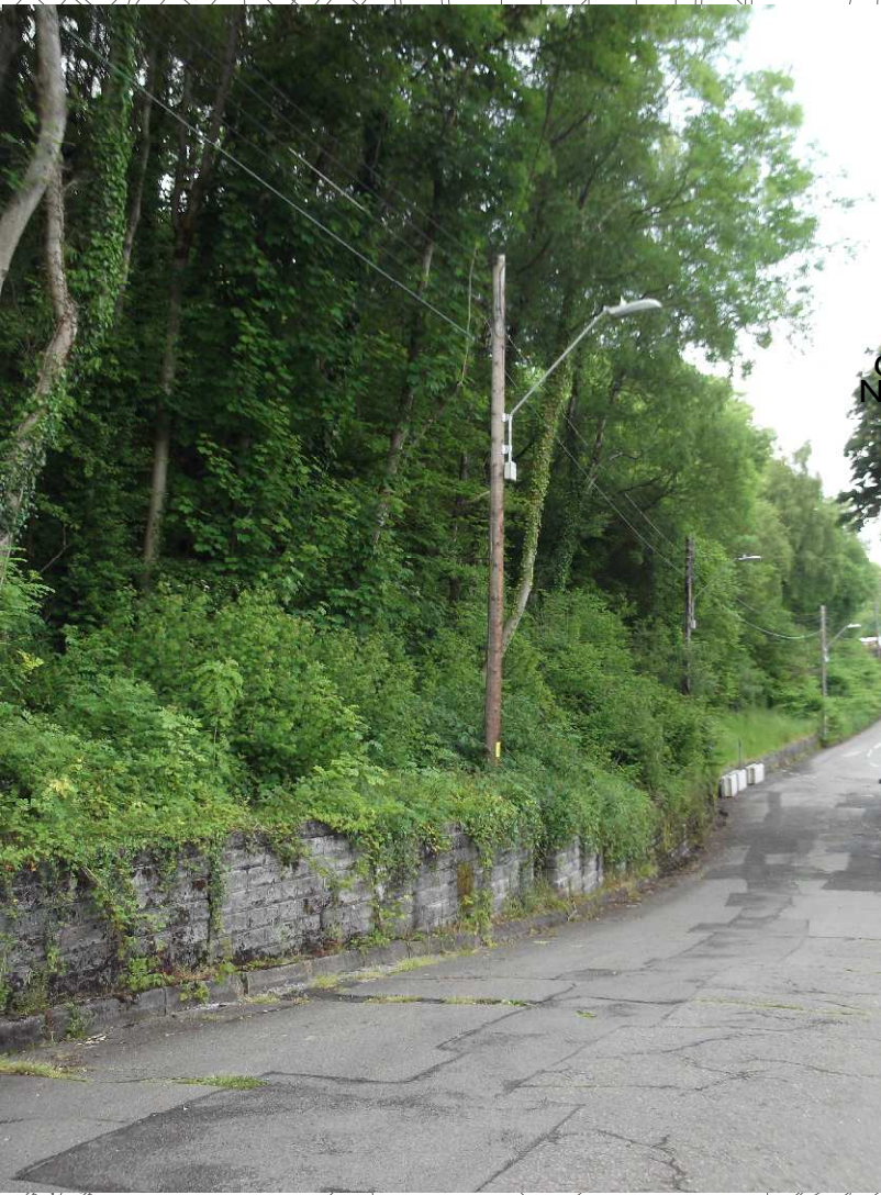
EAST END OF GRAIG ROAD, HEAVILY OVERGROWN, WET AND BULGING
