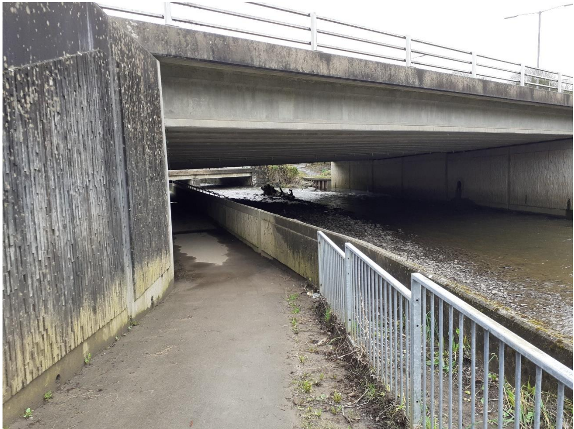
Image 4 – Footpath wall where the river Dulais overtopped, upstream.
