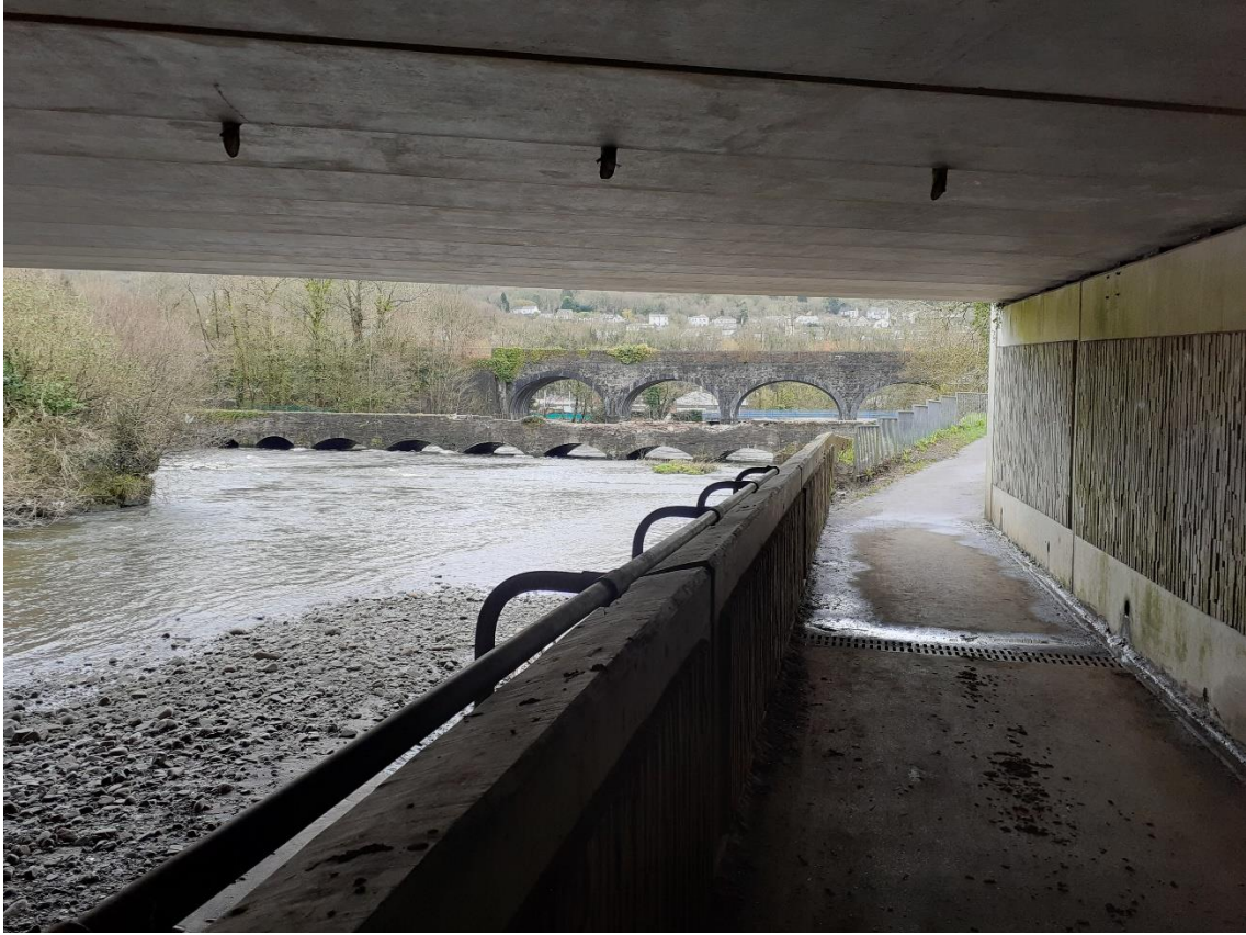
Image 3 – Footpath wall where the river Dulais overtopped, downstream.
